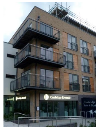
Extensive stained weatherboards at Cambridge Riverside devt
